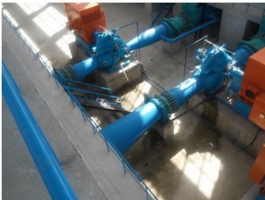
Suvli Pumping Station
