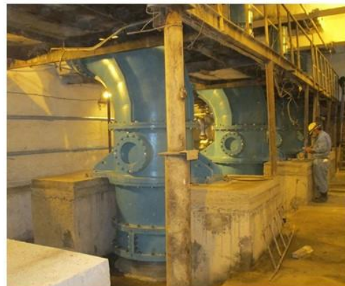
Furkat-1 Pumping Station
