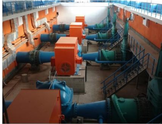
Kizil-Ravat-2 Pumping Station
